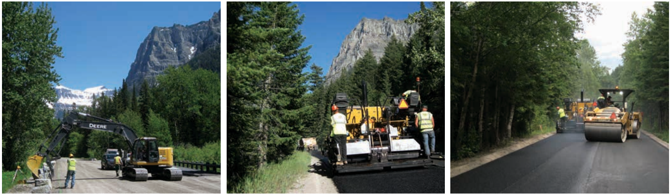
Spring road maintenance is a common, and costly, expense in Glacier National Park. Photos courtesy of NPS.
