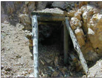
Collapsing timbered adit
