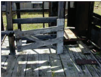
Rotting wooden shaft cover
